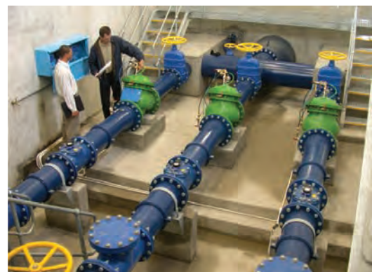
Above: External view of the Khayelitsha pressure management installation, (© City of Cape Town); Khayelitsha pressure management installation, (© WRP (Pty) Ltd)
