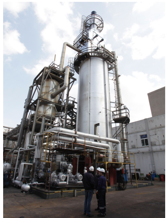
Above: Production unit with installed air cooled heat pumps (© Technology Development Foundation of Turkey)
