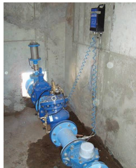
Above: Typical GSM Pressure Logger used in the Web Based data acquisition and display systems (© WRP (pty) Ltd)
