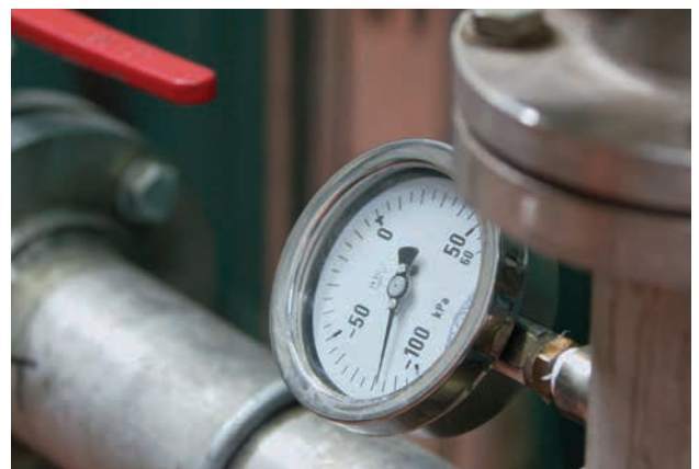
Above: Pressure valve © City West Water
